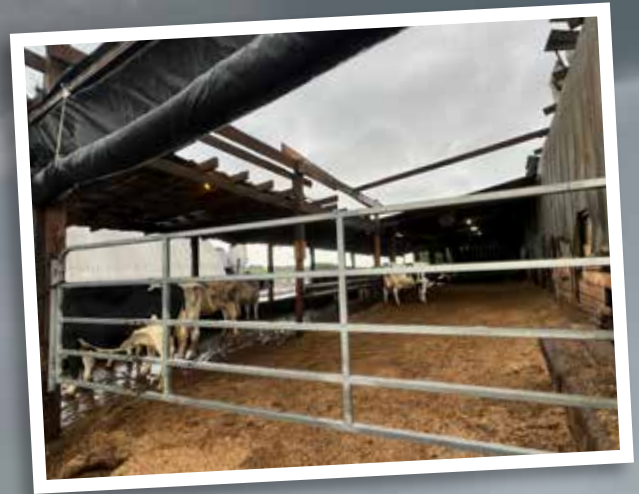
High winds blew off the roof a cow barn. Financial assistance from the Farmers Emergency Fund helped purchase new boards, tin, and building materials.
